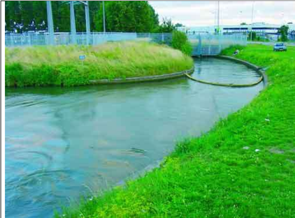
Figure 4 General view site accident. The swirls at the surface are a clear indication of the location of the threshold.
