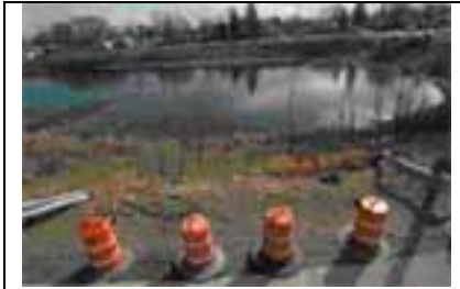
Coby Copeland's car broke through this guardrail at the entrance ramp to U.S. 35 at Gettysburg Avenue.
